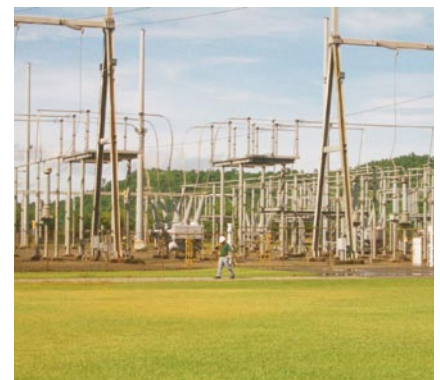
Associated 275kV Switchyard
