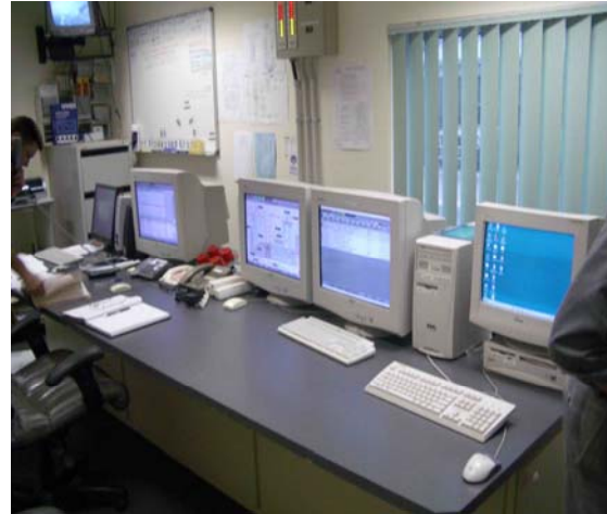
Main Control Room DCS Consoles
