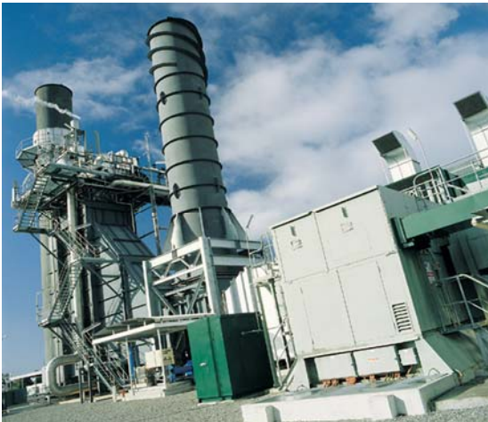
40MW KMK Cogeneration Facility
