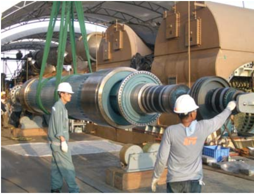
590MVA GE Generator Field Winding
