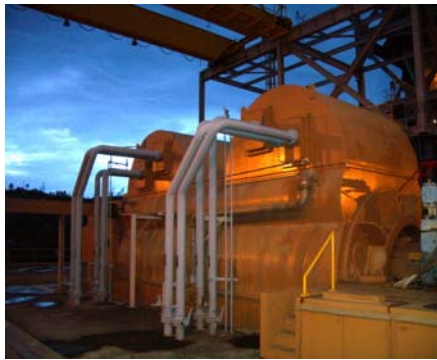
Quezon PS 470MW GE Generator
